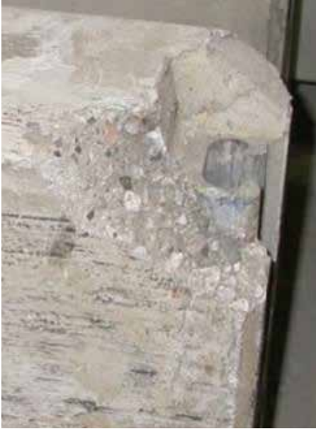
Common Damage: Broken Corner Close to the Y Profile
