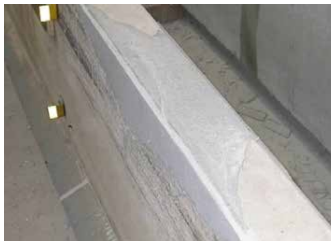
Location of damage after the repair
