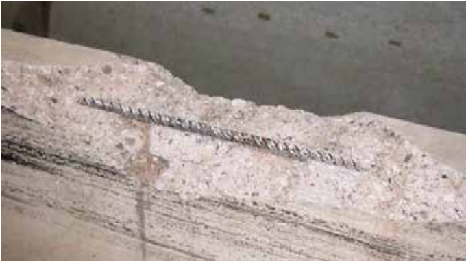
Appearance of damage
